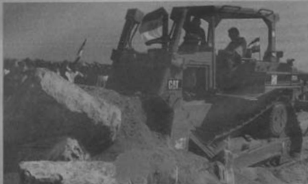
President Rawlings using a bulldozer to clear some concrete slabs and sand to signal the beginning of work on the project.
