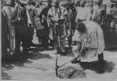
• President Rawlings breaking the ground for the commencement of work on the Market Project for Mankessim.
